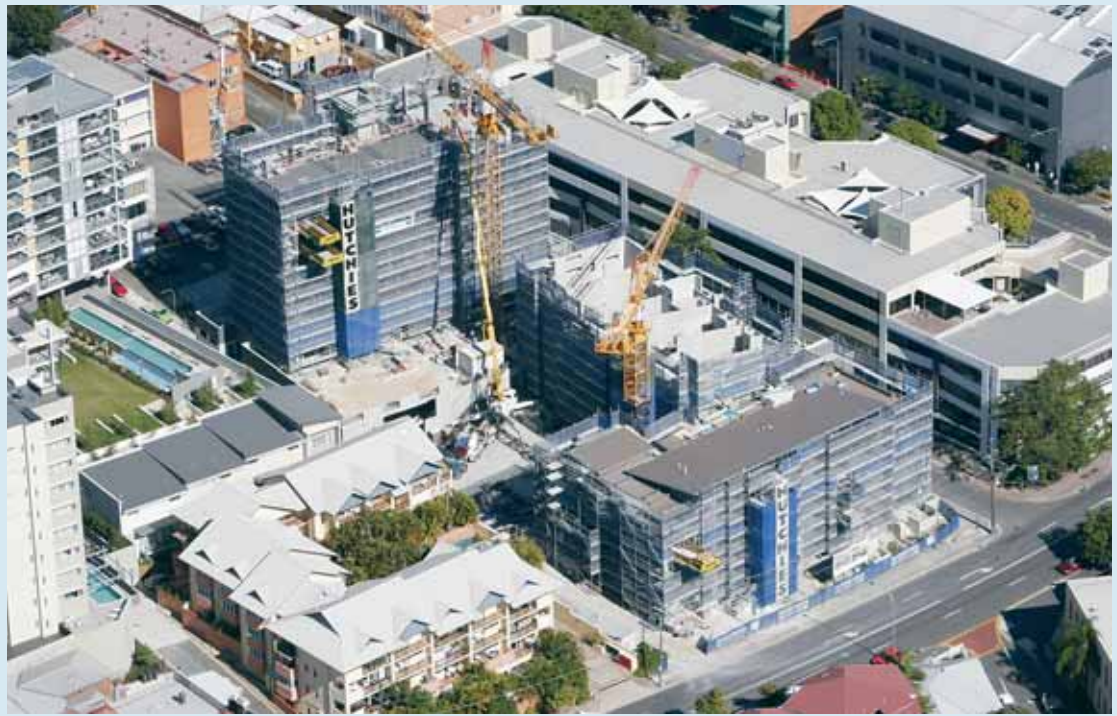
Trilogy Apartments Spring Hill. This is the second stage of the redevelopment of the old Metro Ford site.
